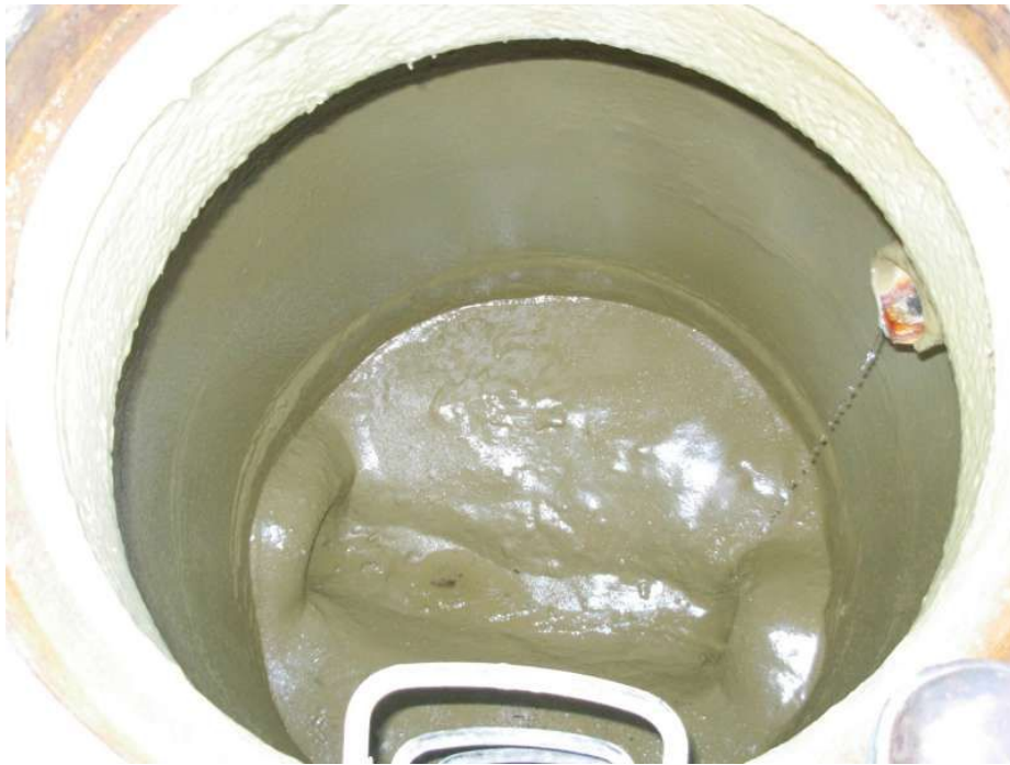
Figure 4 – Example of a manhole with the walls and bottom coated monolithically using a polyurethane liner.
