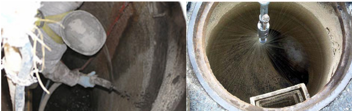
Figures 1 & 2. The figure on the left shows how the ECL is sprayed in place using a shotcrete type nozzle versus centrifugal casting in place which can deliver the ECL at a high velocity that produces good densification without the need for any troweling.
